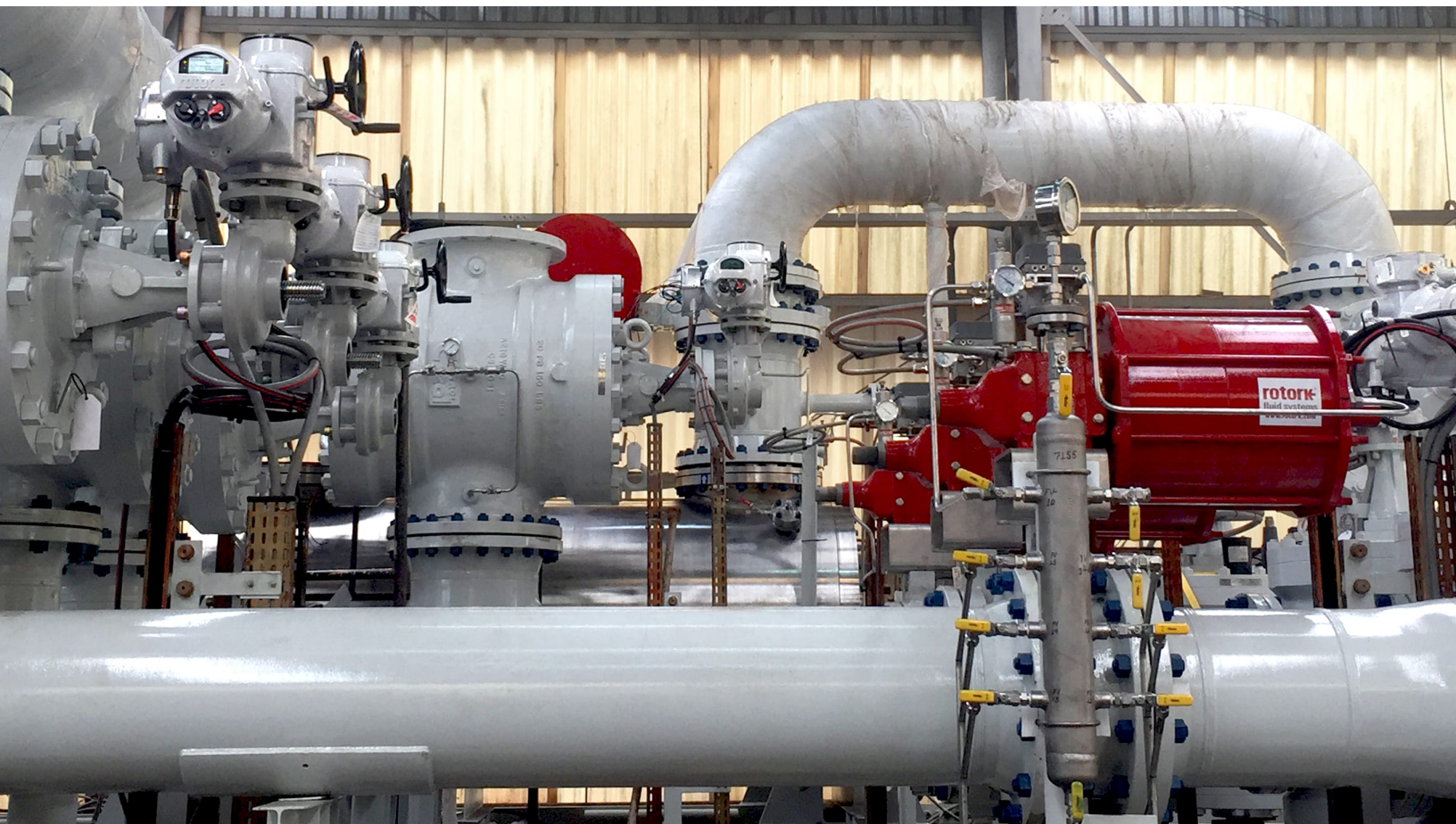
Rotork IQ3 and CP actuators controlling the flow of oil and gas from the FPSO to the metering system.
